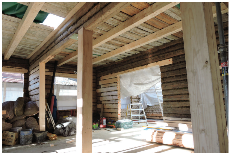
Another room in the ground floor where original ceilings is restored. The floor thickness is about 40 cm, with double crossed floor joist. Technical instalations will fit in between, and the rest will be filled up with cellulose fiber insulation
