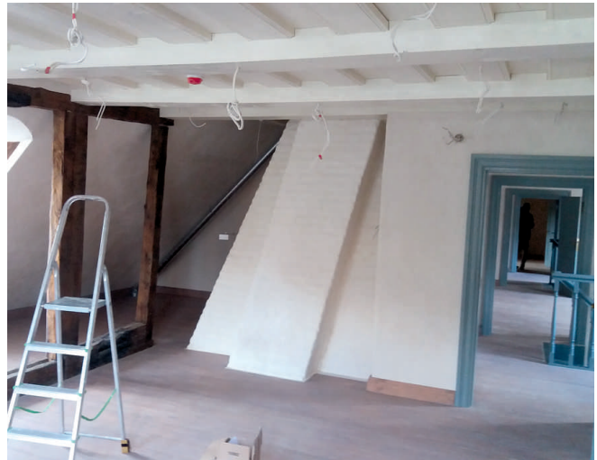
After the rebuilding reconstruction. The cold porches incorporated with the heated and usable premises
