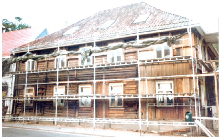
This photo was taken during the work in 1984, and we can see the main part to the left with log walls, and the frame work section to the right. A painted window on the wall in the framework section, to give balance in the facade, is visible in first floor to the right
