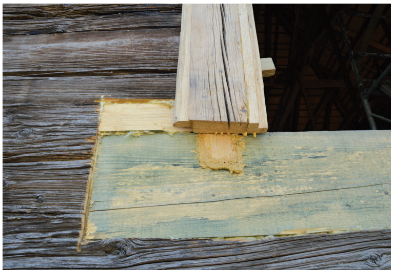
Inappropriate restoration of window frames 2017
