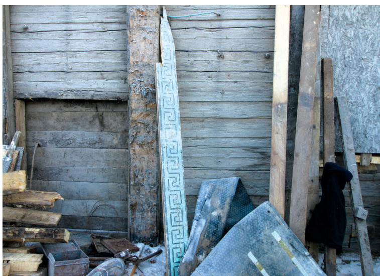
Profile cut of the balcony, damaged fasteners of the walls and board from the vaulting 2017
