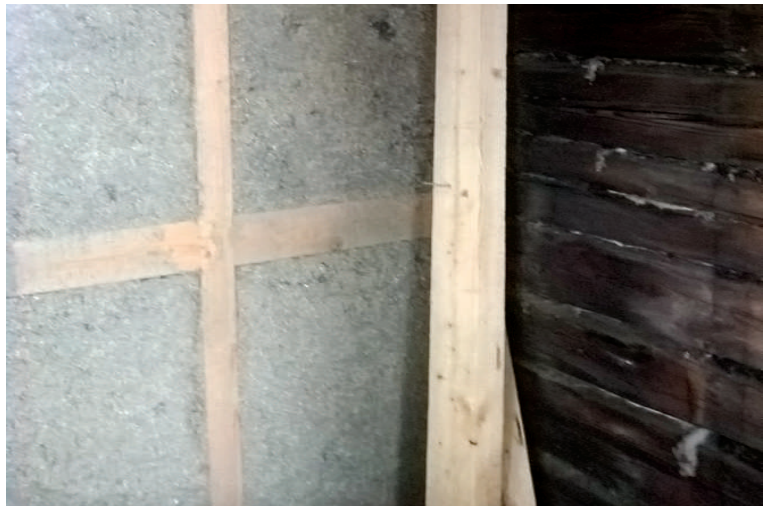
The external vestibule's framework was insulated with 150 mm of wood fiber blown directly on the frame. Photo in 2018, Hanna Elo
