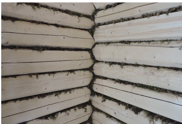
In between the logs we put wet moss ( Hylocomium splendens ) as tradition. This is absolutely the best material for this purpose, and is used all over Norway, Sweden and Latvia. The roof insulation will be put in a rafter construction on top of the ceiling
