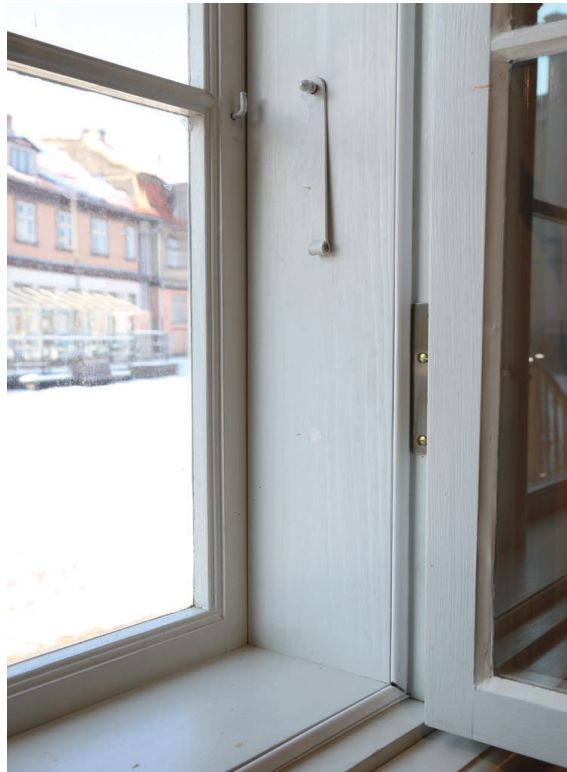
The restorable window with the applicable sealing parts in it – rubber sealing gums and the window glazing with a putty appliance in the external sashes 12
