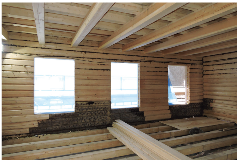
The roof insulation will be put in a rafter construction on top of the ceiling
