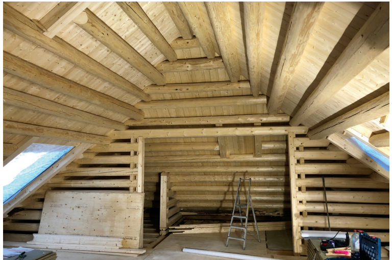
Inside to rooms in ground floor, where we see original ceilings and log walls. The ceiling joists and part of the walls had to be made new
