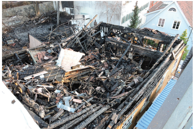
A sad view down in the fire plot, where the roof construction has burnt and fallen down on first floor. Pretty horrible chaos! The whole building was close to collapse!
