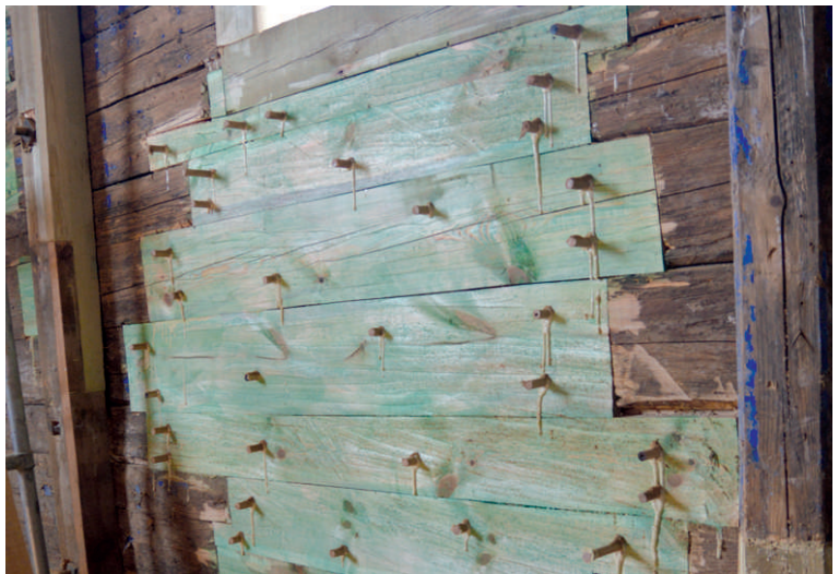
Restoration of wooden wall: implants and partial change of logs 2017 (photo M. Veliulis)
