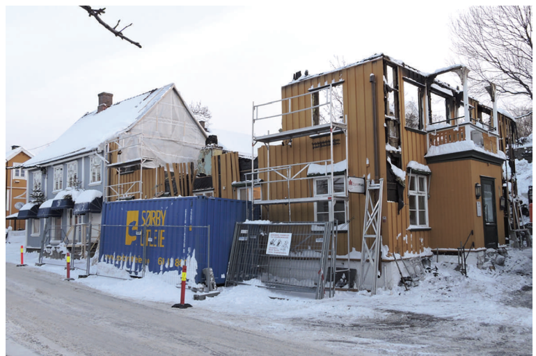
The facades after the fire and the disassembly had started
