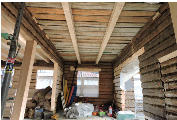
Inside the big hall in first floor, where almost all logs are new. These walls will be visible in the restaurant for several years, until the logs have been compressed and shrunk
