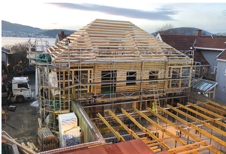
On the 5th. of December 2017 the whole building was back in town, risen up from the ash! The roof construction contains of 850 meters of round logs. In front is the roof of the new kitchen under construction. The kitchen will be moved outside the old building
