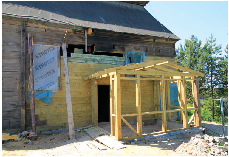
Restoration of wooden wall: implants and partial change of logs 2017 (photo M. Veliulis)
