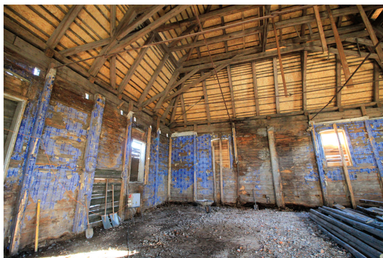
Cleaned the inside of the synagogue before restoration work 2016 (photo M. Veliulis)
