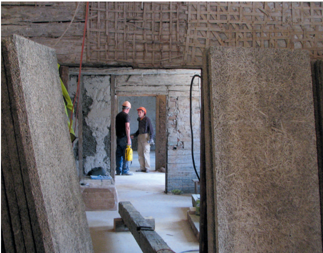
And their dismantled materials which were used in 1973 for reconstruction, including the fibrolite boards
